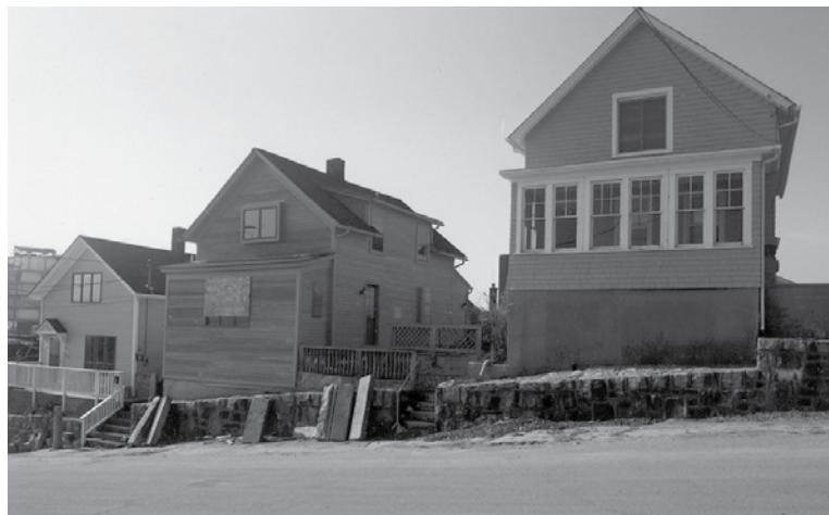
Susette Kelo's little pink house as demolition begins in the area. (Photo by Sylvia Malizia, courtesy of New London Landmarks.)
