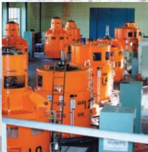
These giant pumps at Detroit's northeastern water plant move treated water from the plant to consumers.
