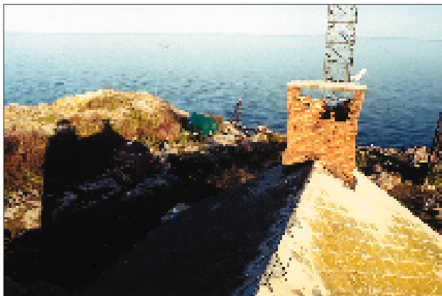
The photo above shows what the roof looked like prior to its replacement. The new roof was made of shingles to replicate the original appearance.
