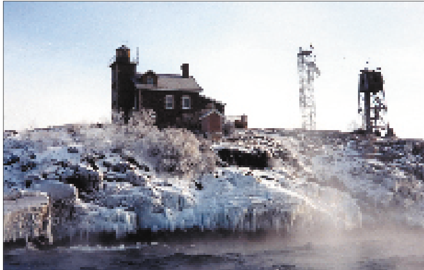
Granite Island lighthouse is located in Lake Superior and is pounded by harsh weather (including ninety-plus mile per hour winds) at least six months of every year. Last November a Nor'easter (storm moving northeast) ripped the island's dock and stairs from rock in which it was embedded.
