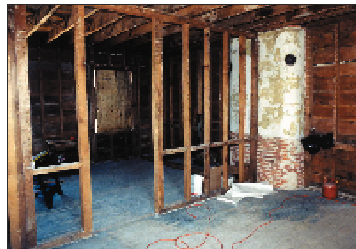
The majority of the lighthouse's insides were gutted, though most of the original floor work was saved and refurbished. This interior photo shows two rooms after being cleared of debris.
