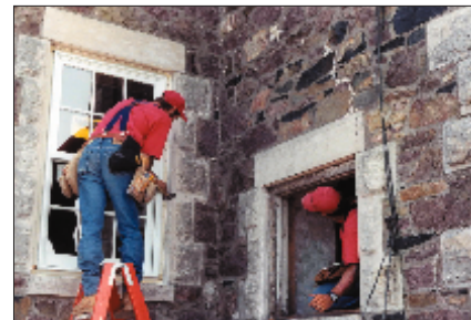
Custom-made windows were installed throughout the lighthouse to replace the originals, all of which were broken by weather or vandals during decades of government ownership.
